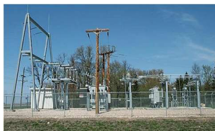
Remote Electrical Substation Wikimedia Public Domain
